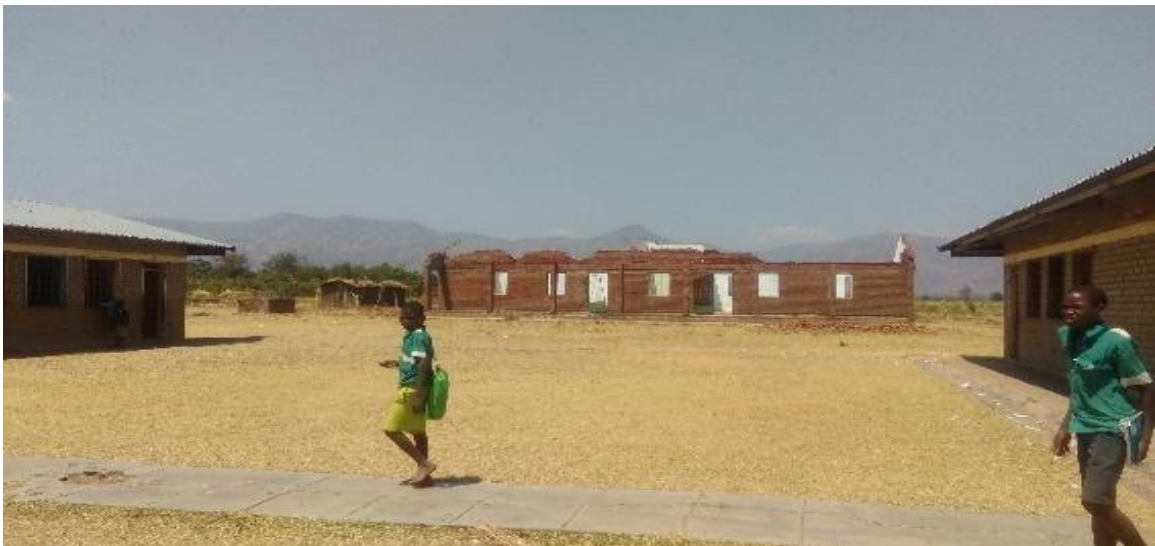
Figure 3: Wolewole school block damaged by strong winds
